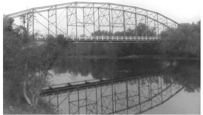
Basso's Ferry bridge over the Tuolumne River, Stanislaus County, California. Built in 1911.)
